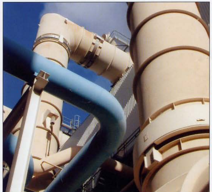
A photograph of the exterior of the Sutton Bridge 800 MW combined heat and power generating facility.
