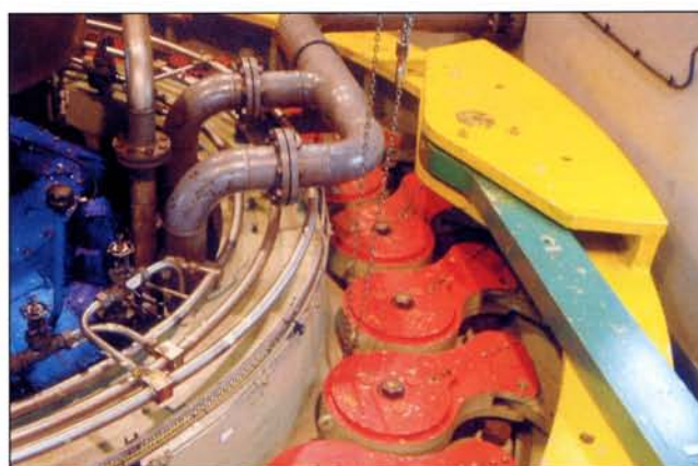
The mechanism of one of the water-powered turbines at Dinorwig. The orange-coloured levers control the ingress of water directed onto the turbine runner.
