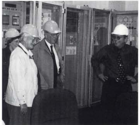
Mr Gregg Bacon of Citigen (right) explains the operation of the CHP control room to a group of Fuellers.
